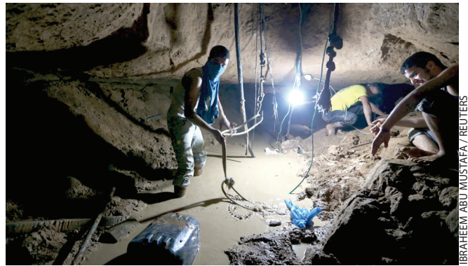
Gazans repair a smuggling tunnel, flooded by the Egyptians, beneath the border between Egypt and Gaza, November 26
